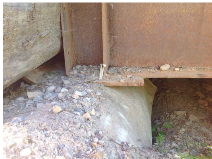
right bank downstream bearing - not fully on log sill - no signs of stress
