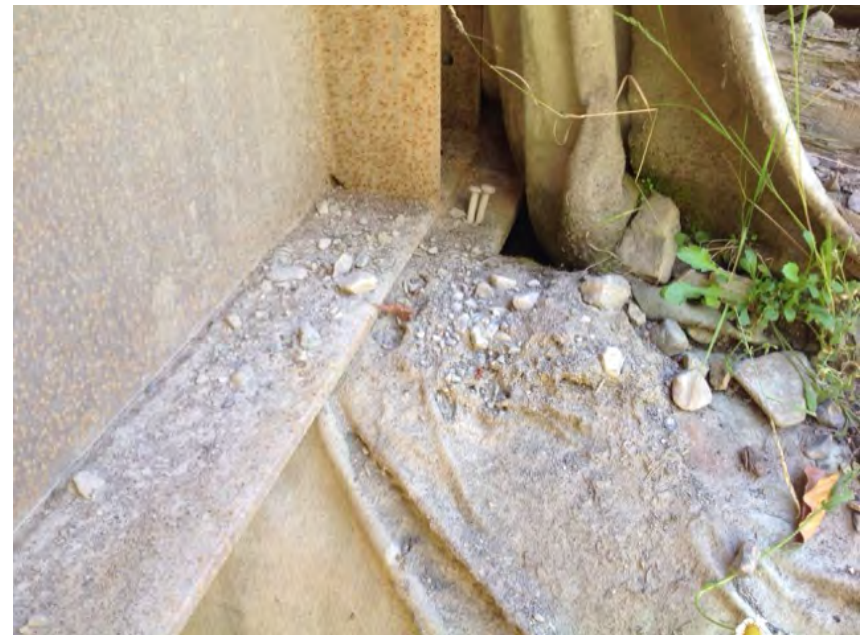
left bank downstream bearing plate barely on log sill - no signs of stress
