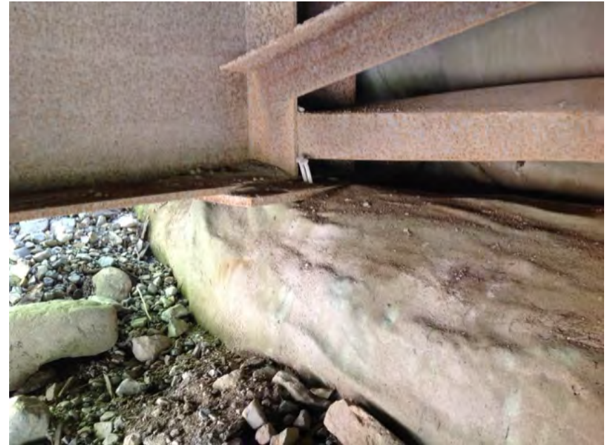
left bank upstream bearing not fully on log sill - no signs of stress
